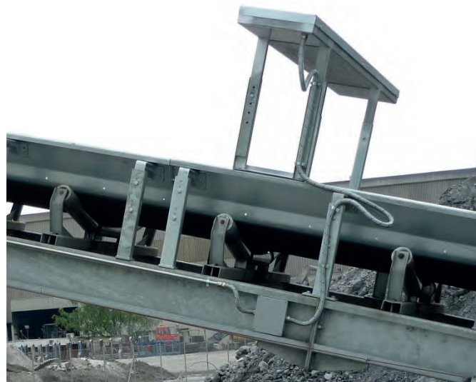
Monitoring of the material carried by a conveyor
